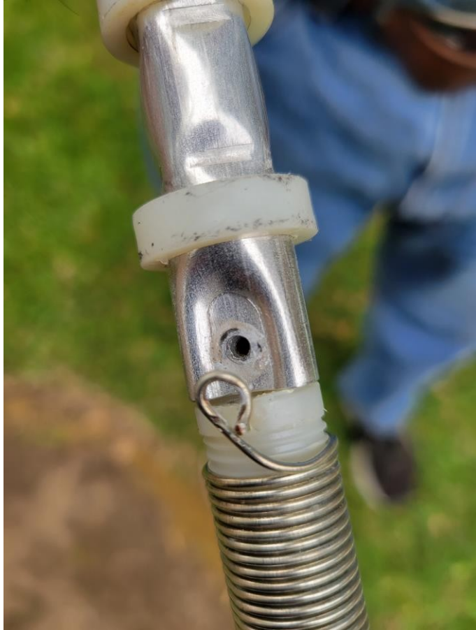
Figure 6 – Corrosion at trap connection before cleaning
