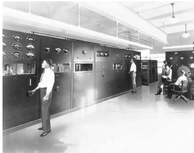
Western Electric's first 550KW transmitter, model 7A, was installed at WLW in 1928 (from The Radio Historian)
